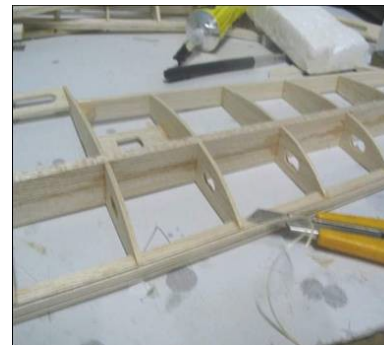
Draw a reference along the S1. Trim and sand to round the leading edge along the lines
